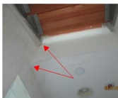
Figure 6: Similar water damage in
