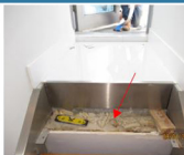
Figure 4: Water damage at stair landing
